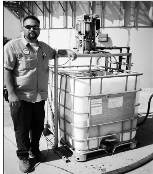
Raudel Juarez, VRSD Operator, insures the polymer system is ready when sludge is transferred to the Geotube®.
