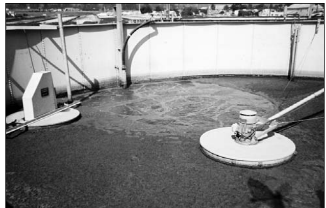
Two large circular tanks operated in batch mode provide alternating aerobic, anoxic, and clarification treatment of the wastewater.
