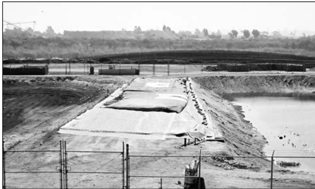
45 ft C x 43 ft L Geotube® is laying on a MCF-1210 ground cover which captures the clear filtrate to flow back to the headworks.
