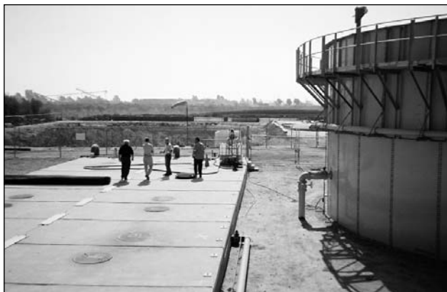
Saticoy Facility showing large septic tank now operating as aerobic digester prior to going to Geotube® containers seen in background.
