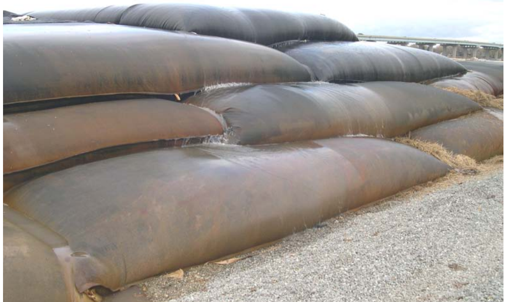
Geotube® containers stacked in a dredging operation at Fox River. Geotube® dewatering containers can be layered like this to increase dewatering volume for the space allotted. For a large project, this can be critical.
