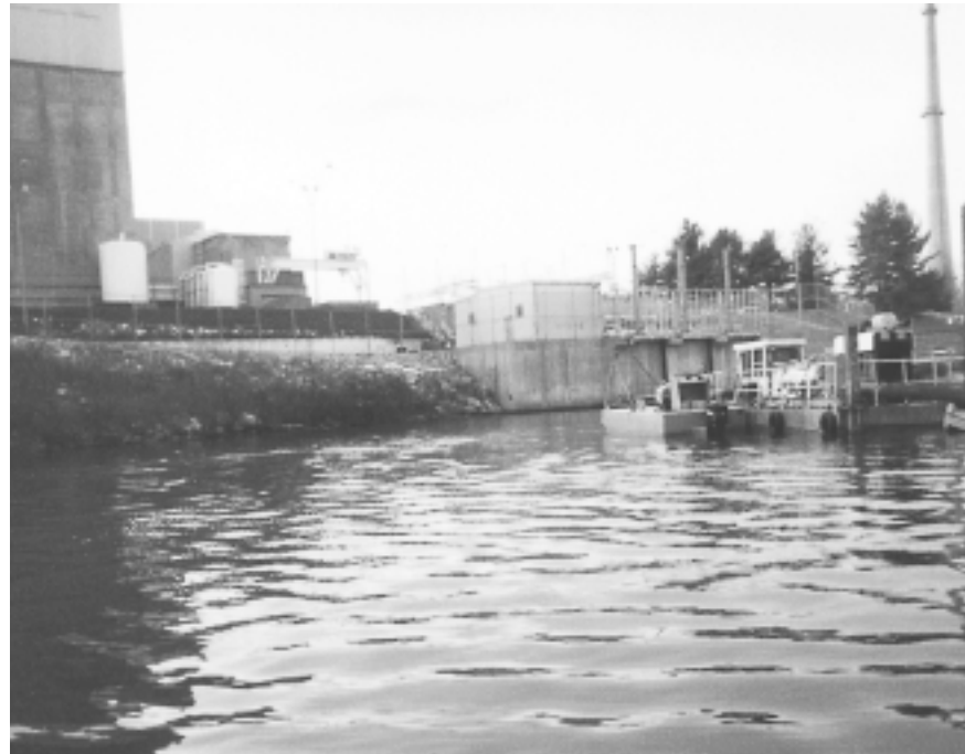
Dredge material pumped out of intake lagoon 2200 LF to field where 12 300" long by 30' circumference Geotube® structures were placed.
