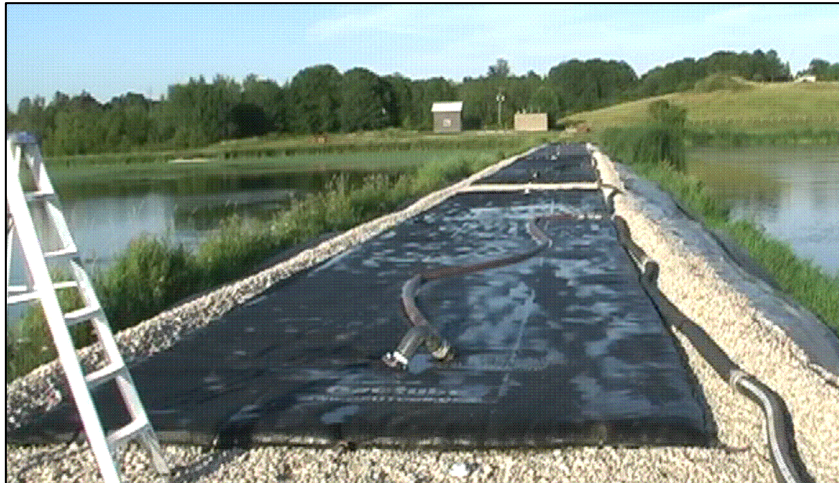
In August 2009, Six Geotube ® units were used to dewater and contain sludge pumped from one of the three sewage lagoons operated by The Municipality of Arran-Elderslie.
