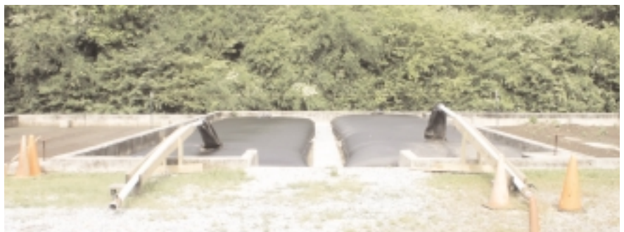
Geotube® containers being filled with solid waste pumped from the digester. Two tubes fit within this drying bed. The city of Eatonton is pleased with the Geotube® Containers.
